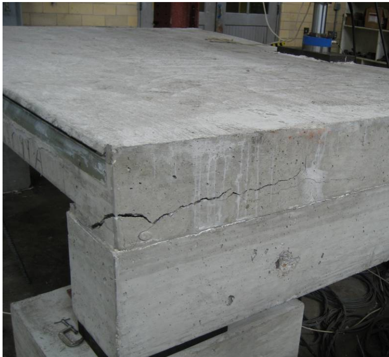
Figure 5.8: Delamination from Support Beams at Northeast Corner of Specimen P0P1
